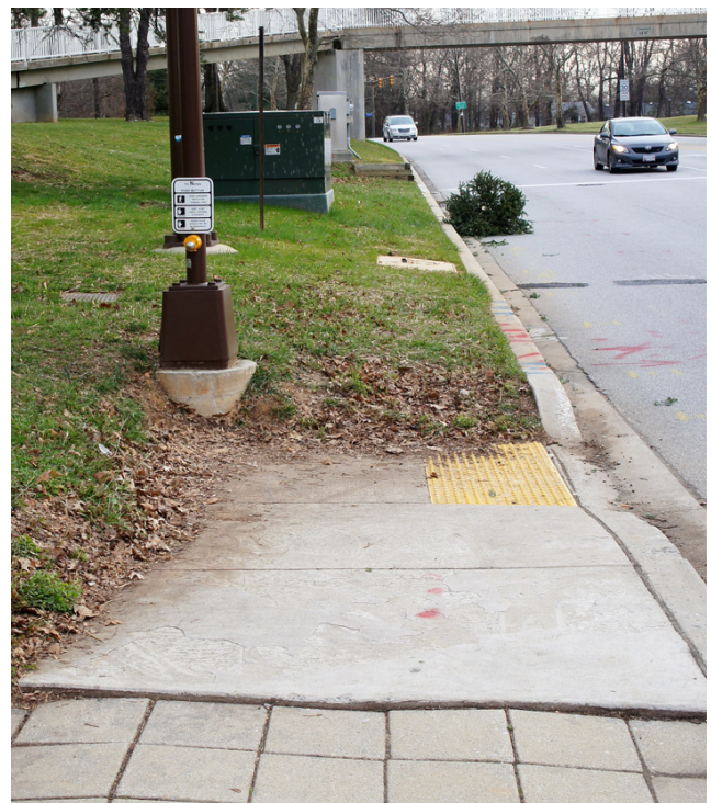
Sidewalk to “no-where” inhibits active transportation (pedestrian and cycling)
